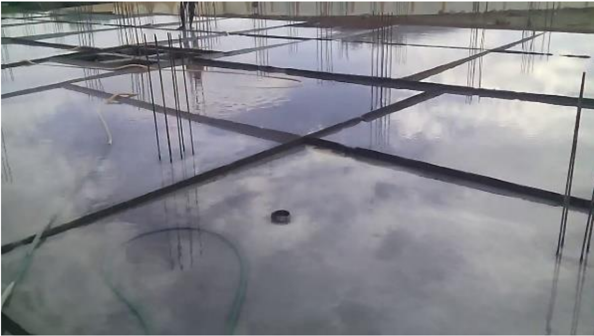
Fig.: Ponding of concrete
