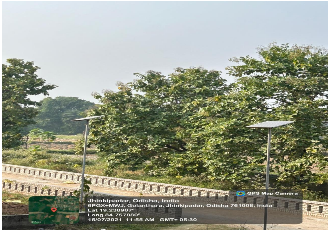
Solar Street Light
